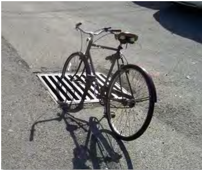
Unsafe Grate for Bicycles - Bike PGH
